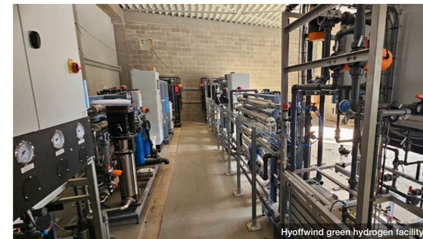
Hyoffwind green hydrogen facility
