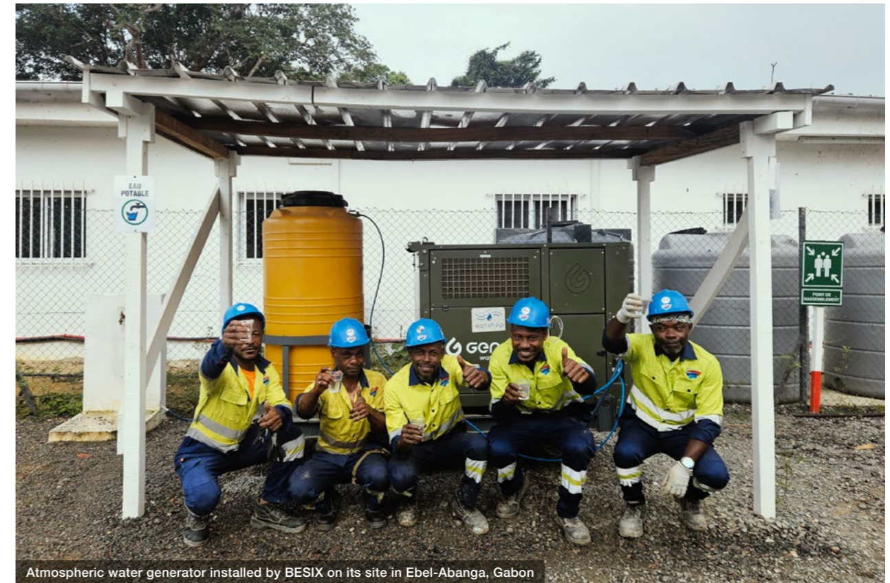
Atmospheric water generator installed by BESIX on its site in Ebel-Abanga, Gabon
